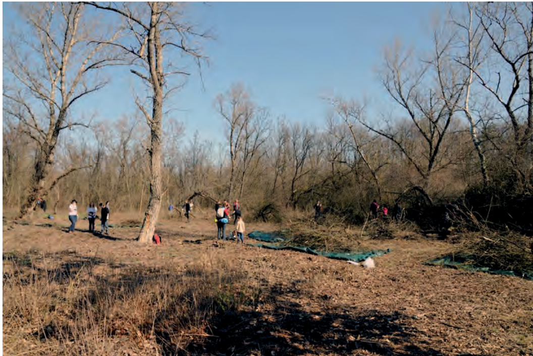
Fig. 10. In the course of habitat management the invasive alien woody species are removed manually. The produced timber is placed on tarp and taken off the grassland to a dirt road on the edge of the habitat. (Photo: Z. Bajor)
